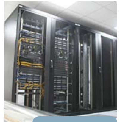
2bm's state-of-the-art server room solution
